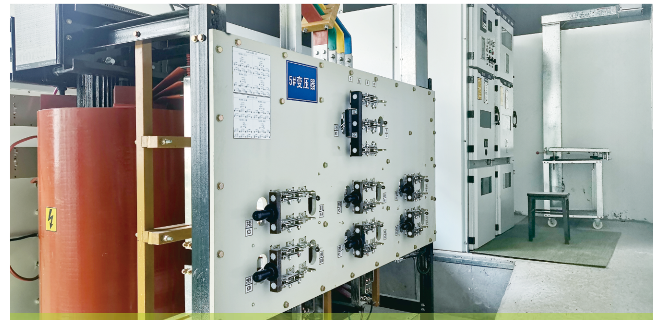
短路设备02 Short Circuit Equipment 02
