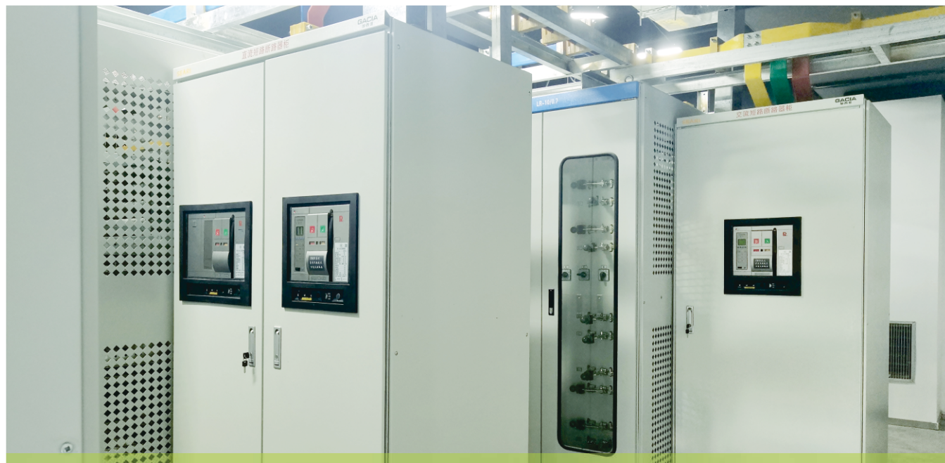
短路设备01 Short Circuit Equipment 01
